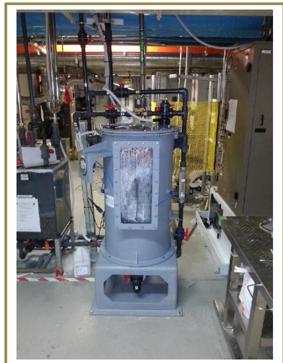
Mini Scrubber Installation for a R&D lab at a local university
