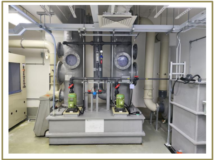
Vertical Two-Stage Scrubber for a manufacturing plant
