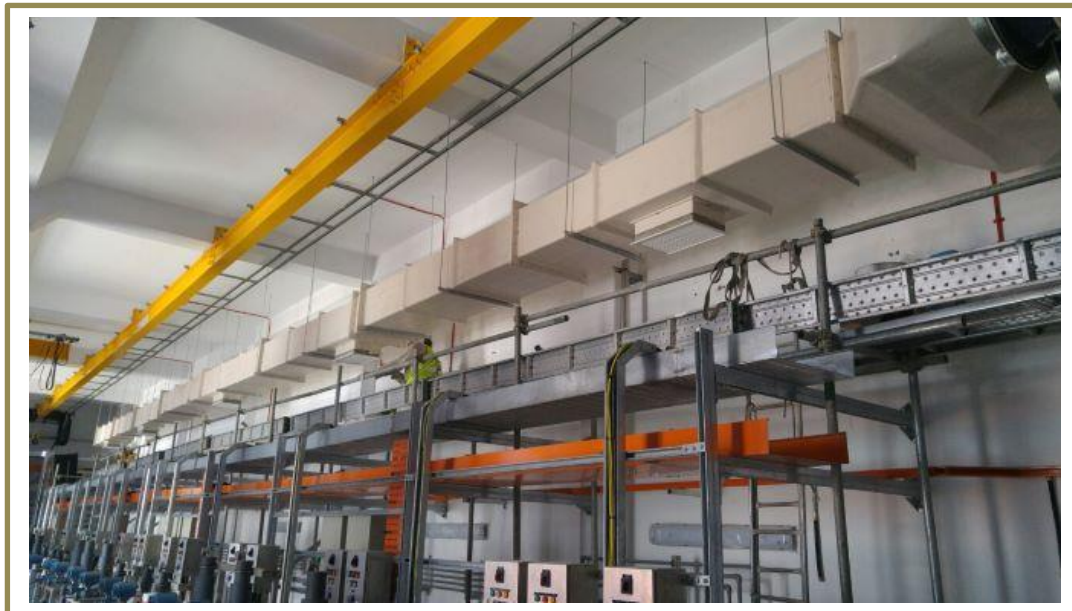
Rectangular ducts for PUB plant
