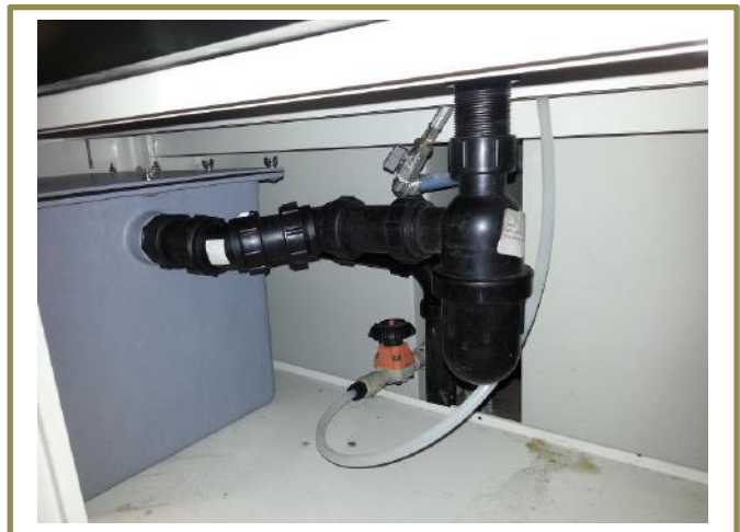
Dilution Tank for laboratories of a local polytechnic
