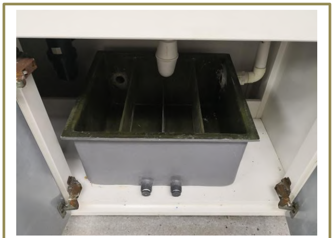
Dilution Tank for a hospital (opened to show interior)
