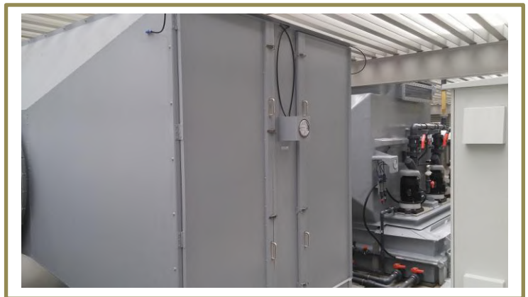
V-Bank ACF with Wet Scrubber Installation for a local university
