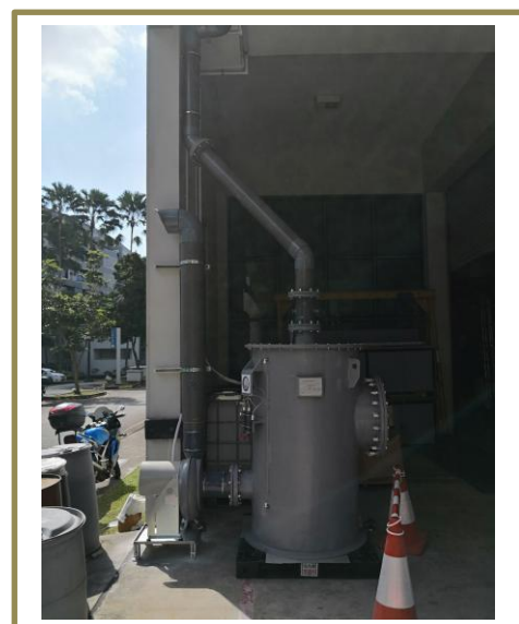
Activated Carbon Filter Installation for odour and toxic gases abatement
