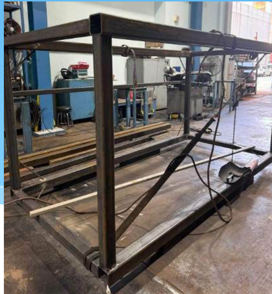
Galvanised Steel Structure
