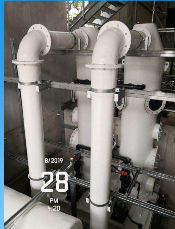
Vertical Counter-Current Scrubber System
