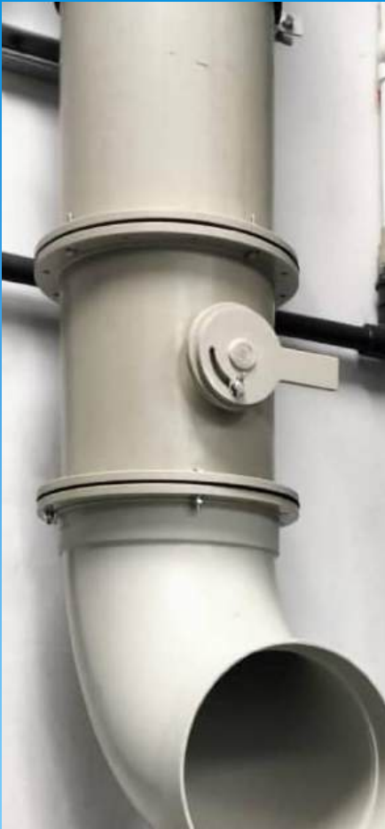
PP Damper and Ducts
