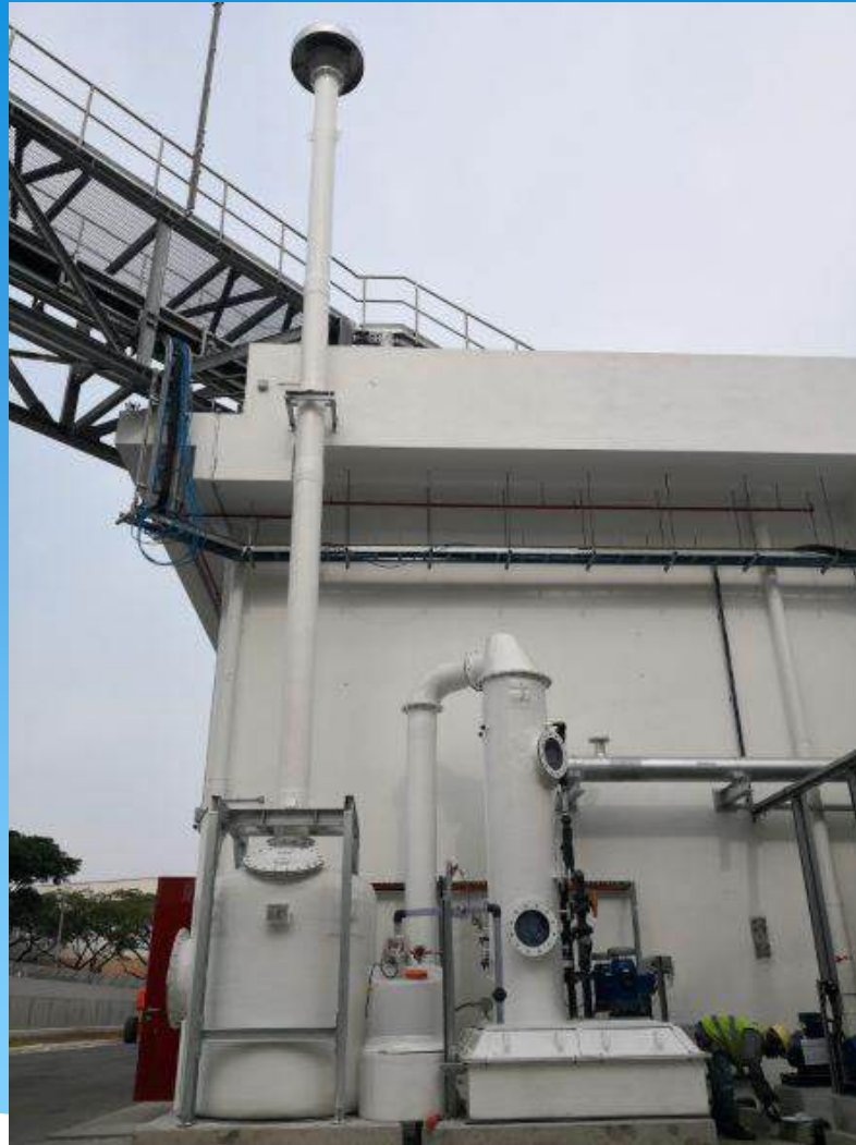
Combined Systems for a waste treatment plant
