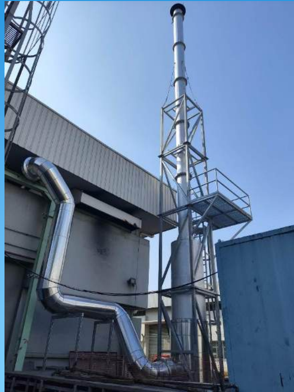
Steel Exhaust Ductings with Silencer and Certified Structure
