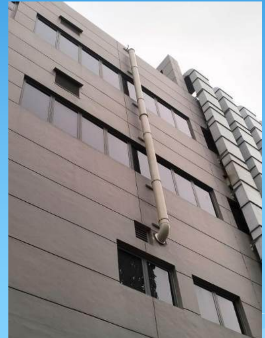
PP Exhaust Ductings and Stack
