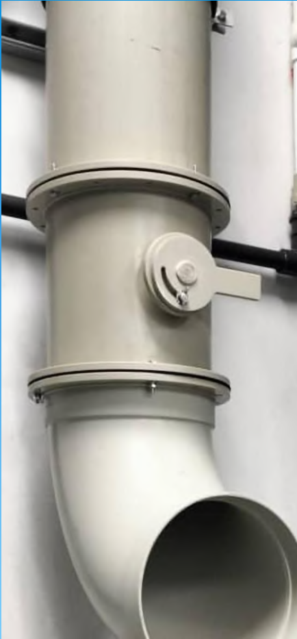
PP Damper and Ducts
