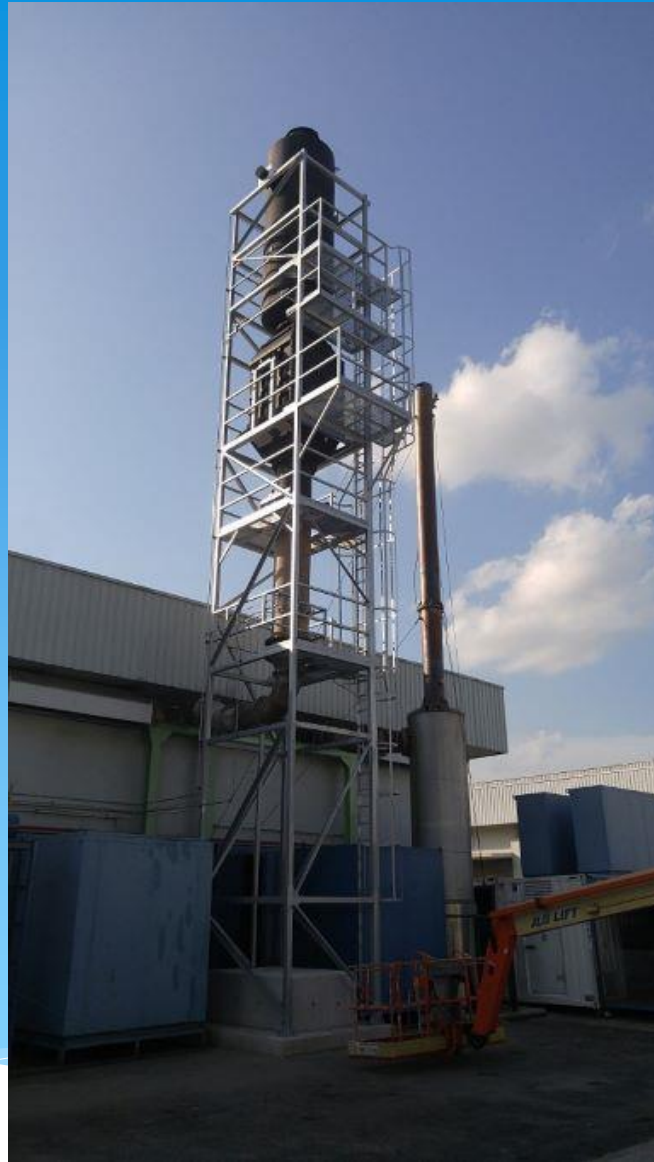
Selective Catalytic Reduction (SCR) System - Supply, install, test and commission
