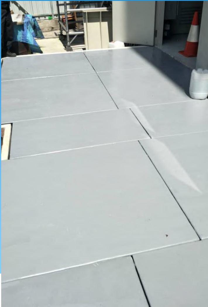
FRP-lined Steel Skids
