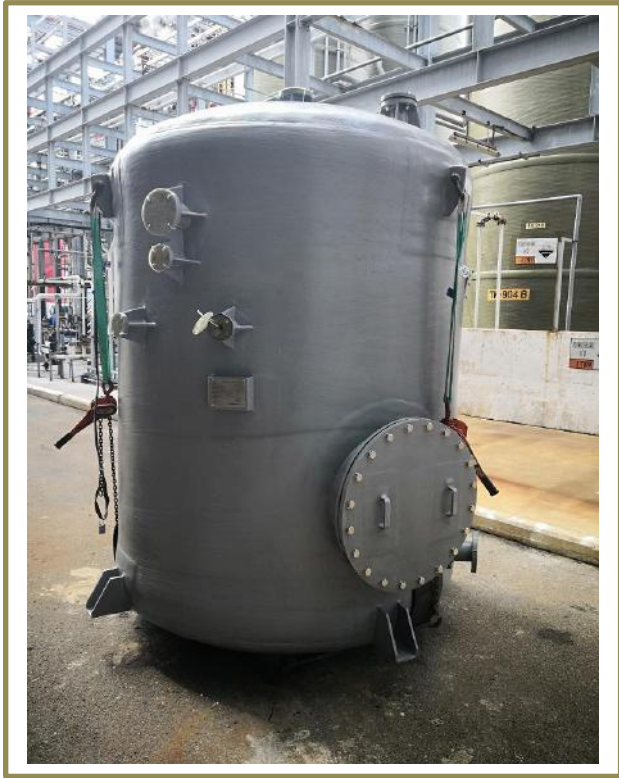
Chemical decomposer tank
