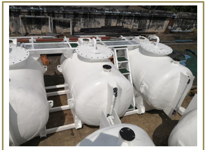
Sodium Hypochlorite storage tanks incorporated with skid, ladder, platform and foldable hand rail
